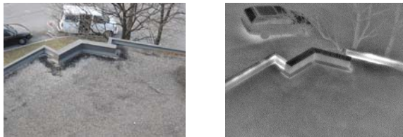
Figure 3: Convection heat loss at wall corner/flat roof perimeter detail. Masonry brick wall appears to be wet, due to moist warm interior air ex-filtrating through exterior wall system.
